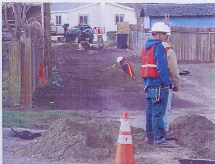
ABOVE: Two NPL crews installed 5,752 feet of replacement main in just over nine days, averaging more than 600 feet each day.
