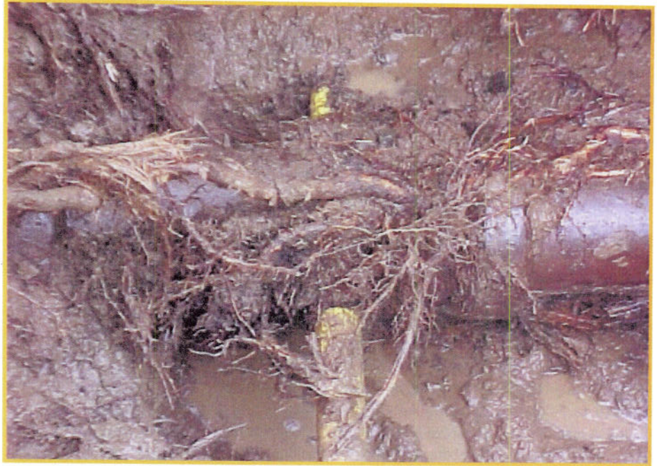
A breached sewer line is called a “cross-bored line,” and can occur even with conscientious pipeline installation. Photo courtesy of the Minnesota Office of Pipeline Safety
